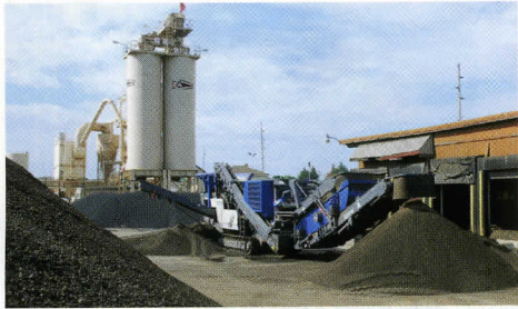
ABOVE: Plant Manager Chuck Royer said integrating the Mobirex MR 110 Z crusher into the Tri-County Asphalt Materials operation was relatively easy.
